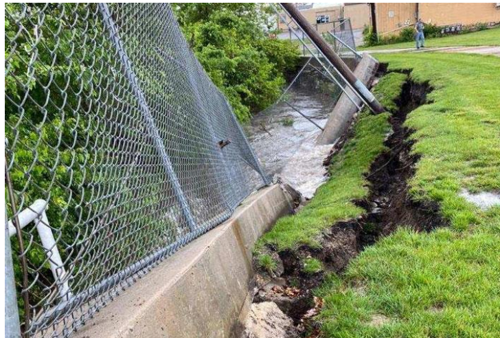
Figure 3. Rock Creek Channel Wall Failure (Shawnee Mission Post 2020).
