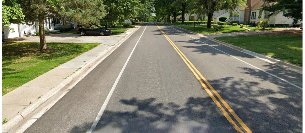
Figure 6.8 - Existing Sidewalk Condition along Lamar Avenue - Sidewalk on Only One Side of the Road and Inadequate Distance from Moving Traffic
