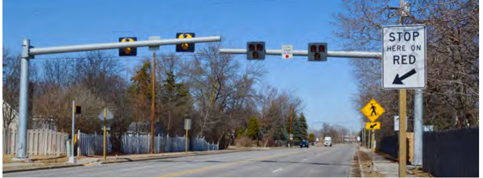
Figure 6.5 - HAWK Beacon for Mid-Block Pedestrian Crossings
