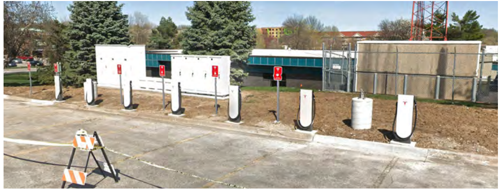
Figure 6.14 - Charging Stations Located at Hy-Vee in Mission
