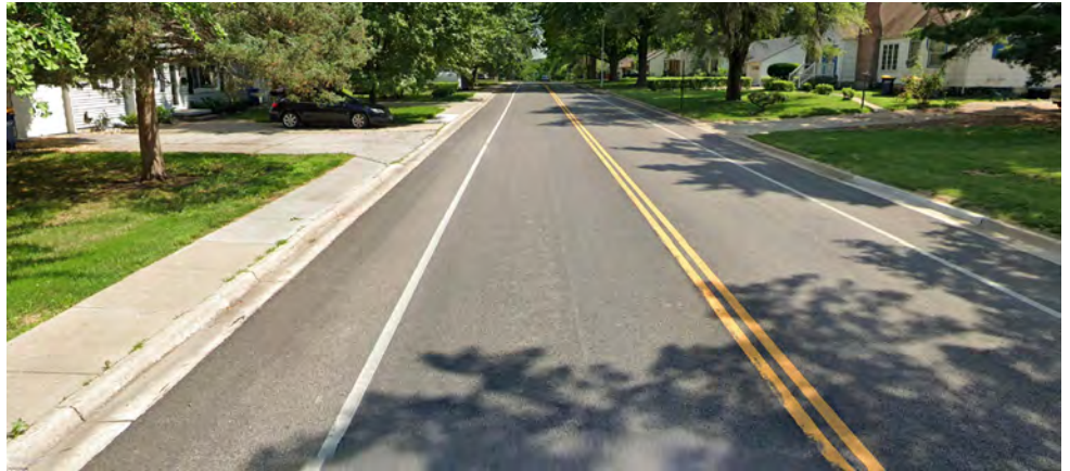
Figure 6.8 - Existing Sidewalk Condition along Lamar Avenue - Sidewalk on Only One Side of the Road and Inadequate Distance from Moving Traffic
