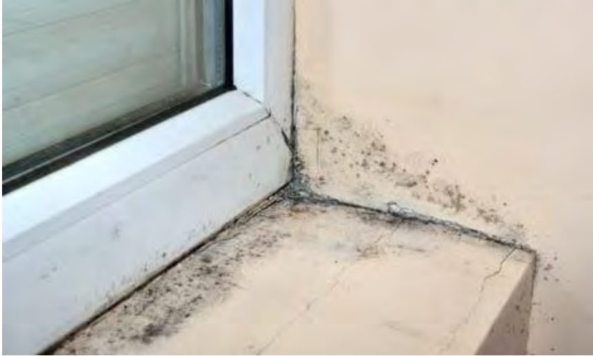
HOW WINDOW CONDENSATION CAUSES DAMAGE
