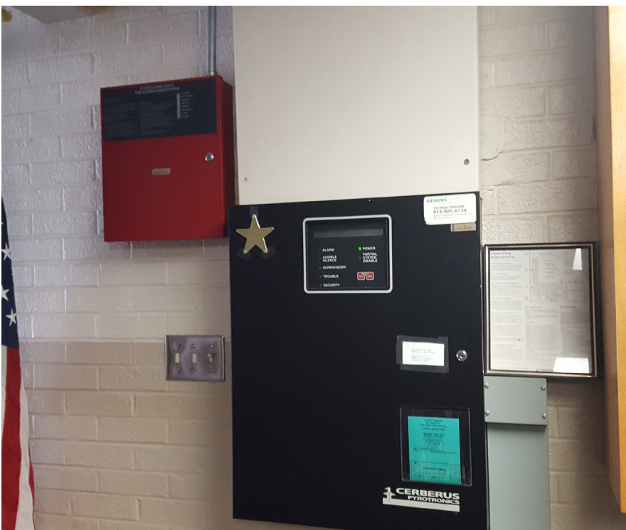
Main fire alarm control panel for outdated system
