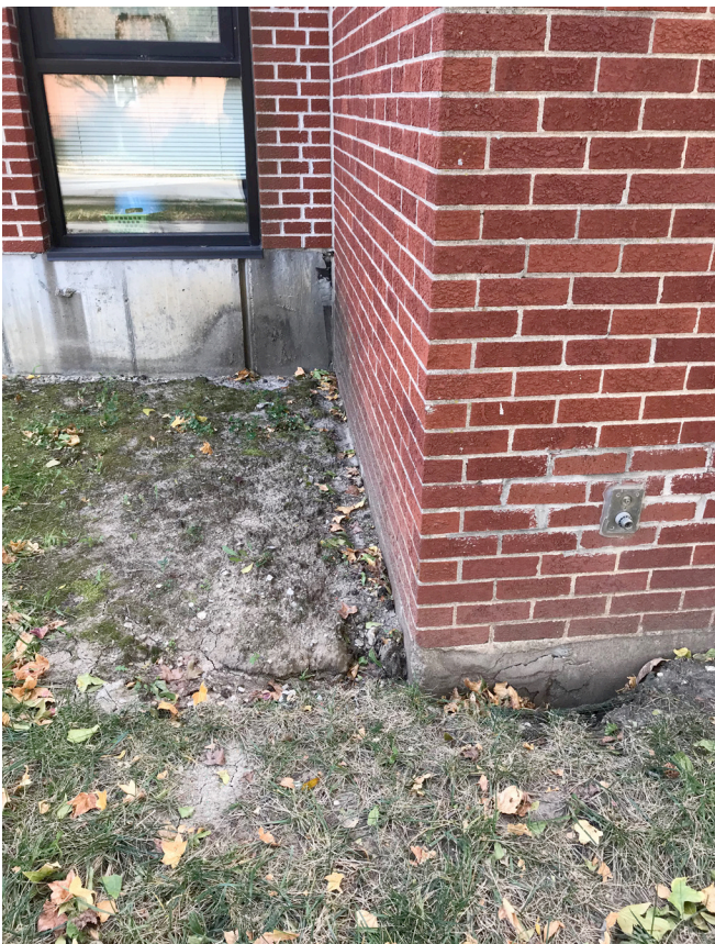
Exterior building: maintenance issues at brick and foundation walls.
