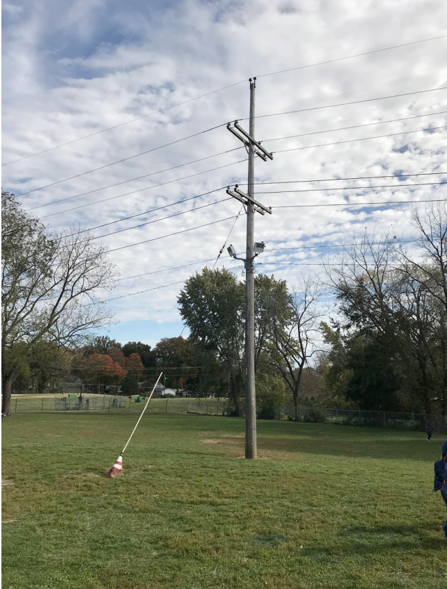
Overhead powerlines running through the playground areas. Guy wires are a tripping hazard.
