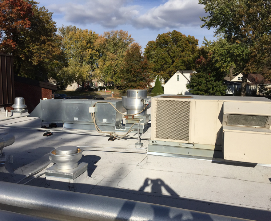
Distance from exhaust outlet to outside air intake should be a minimum of 10 feet does not appear to be
