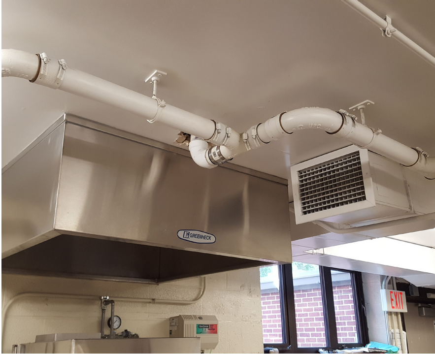
Sanitary vent piping near kitchen dishwasher
