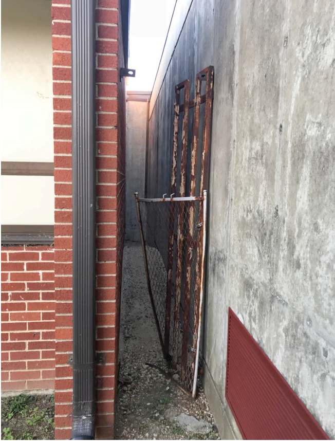
Exterior building: maintenance issues at brick and foundation walls.
