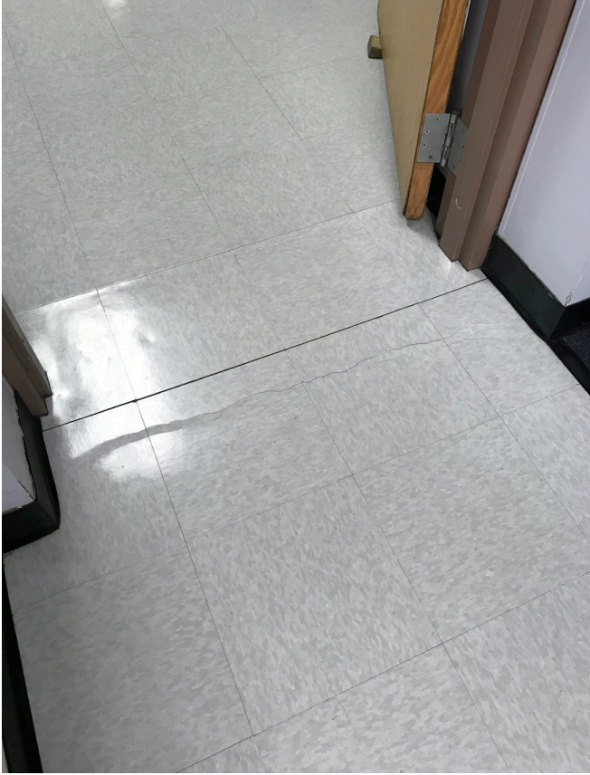
VCT flooring with cracks and unlevel surface for walking.
