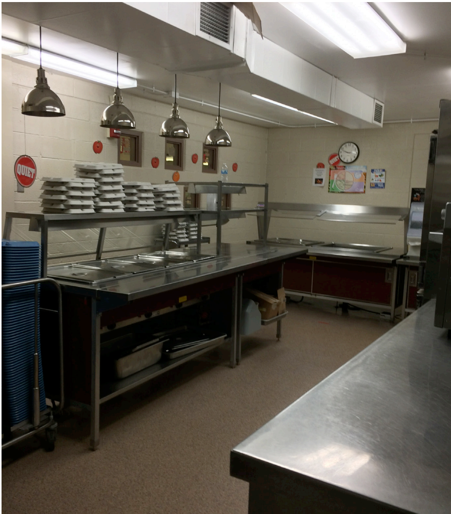
Small kitchen/serving area. Exposed ductwork directly over food areas.
