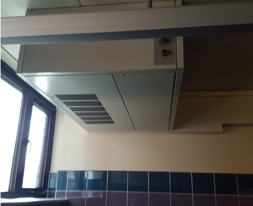
HVAC unit in restroom - accessible to students
