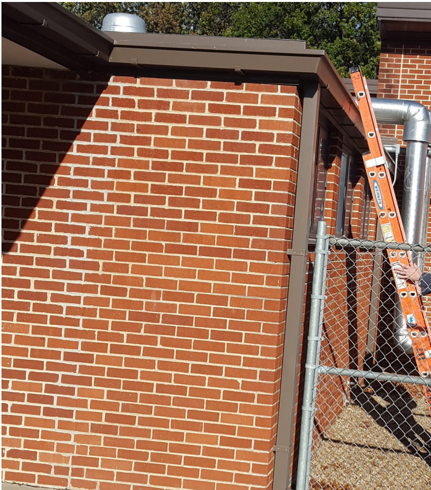
Roof Access is not permanent
