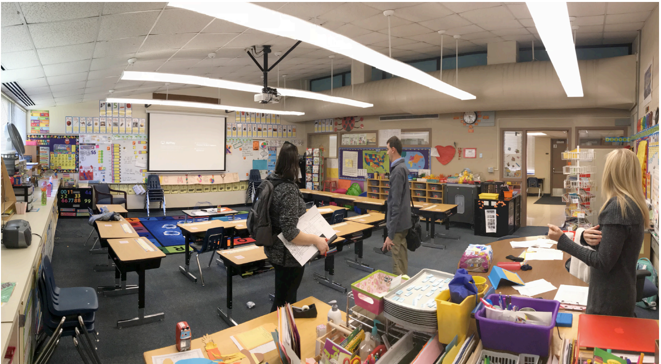
Small classrooms (709 s.f.) with traditional desks. Need different furniture types to allow for various teaching instruction. HVAC moisture problem is causing drooping ceiling tiles. High clerestory windows are covered up and large mechanical ductwork also blocks the clerestory windows.
