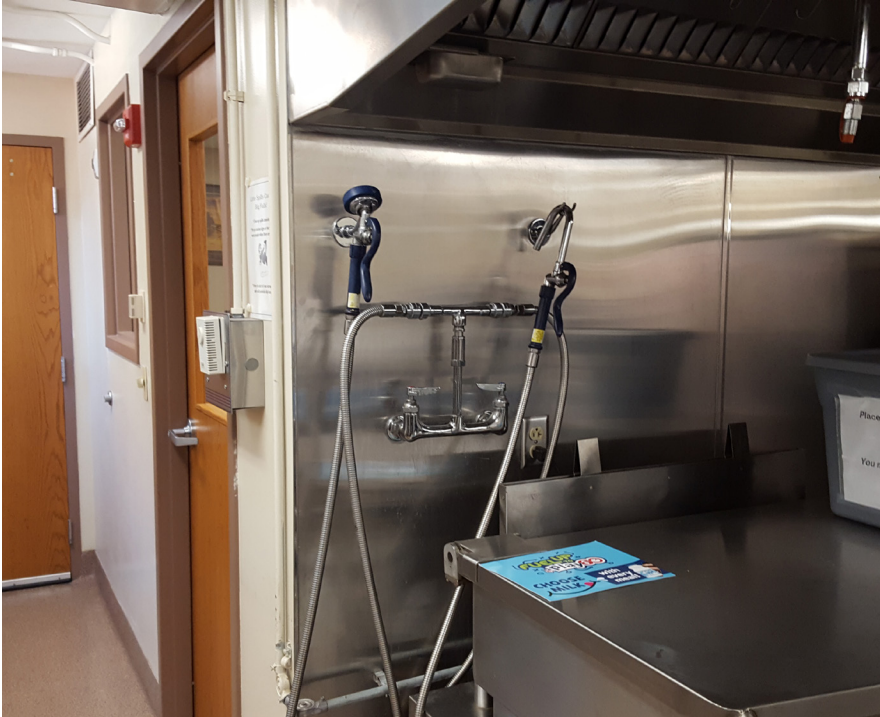
Thermostat near cooking line could cause false operation
