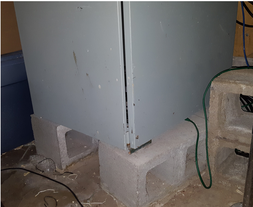
Data rack on blocks in basement that floods
