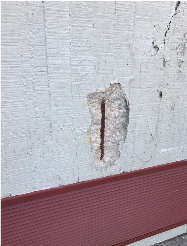
Concrete surface deterioration due to moisture issues.
