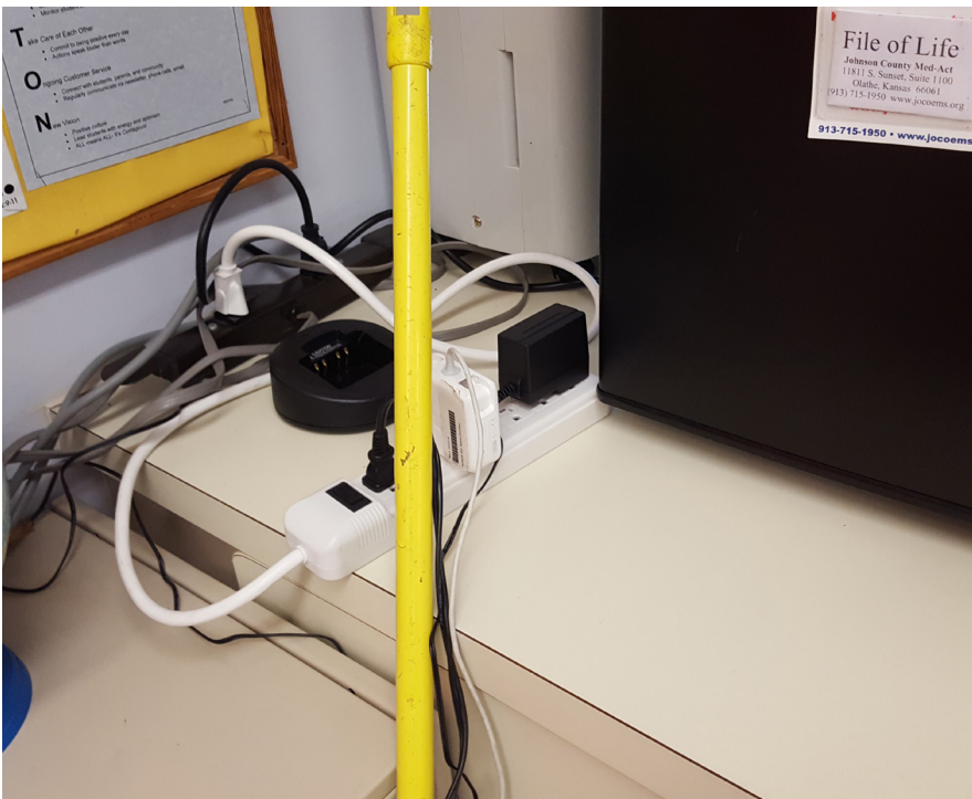
Insufficient electrical outlet quantities
