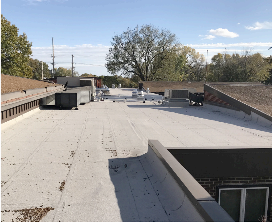
Gravel at ballasted roofs is washing away. No permanent roof access.
