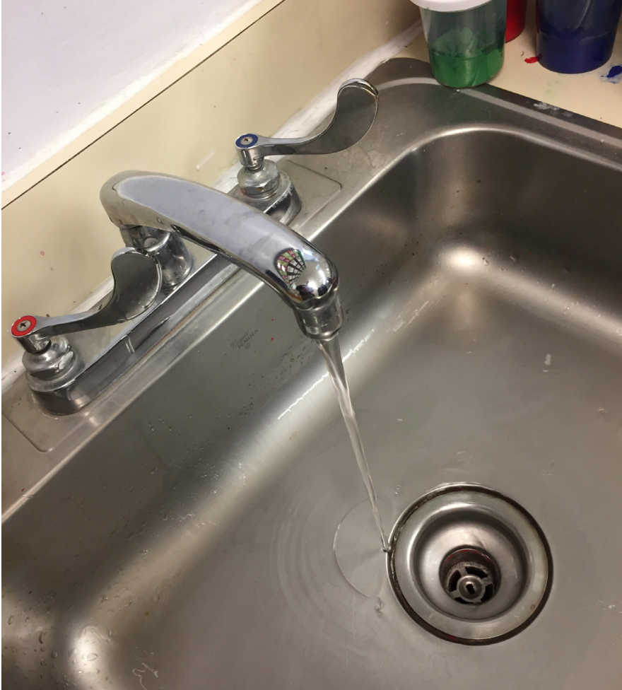
Low pressure for hot water supply from classroom sinks
