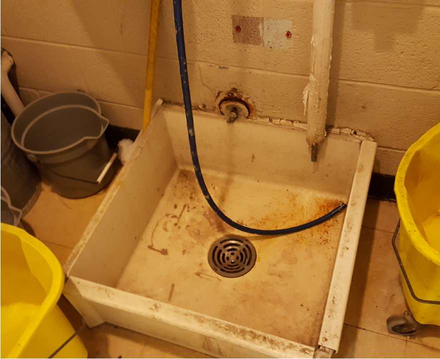
Mop sink deteriorated recommend replacement
