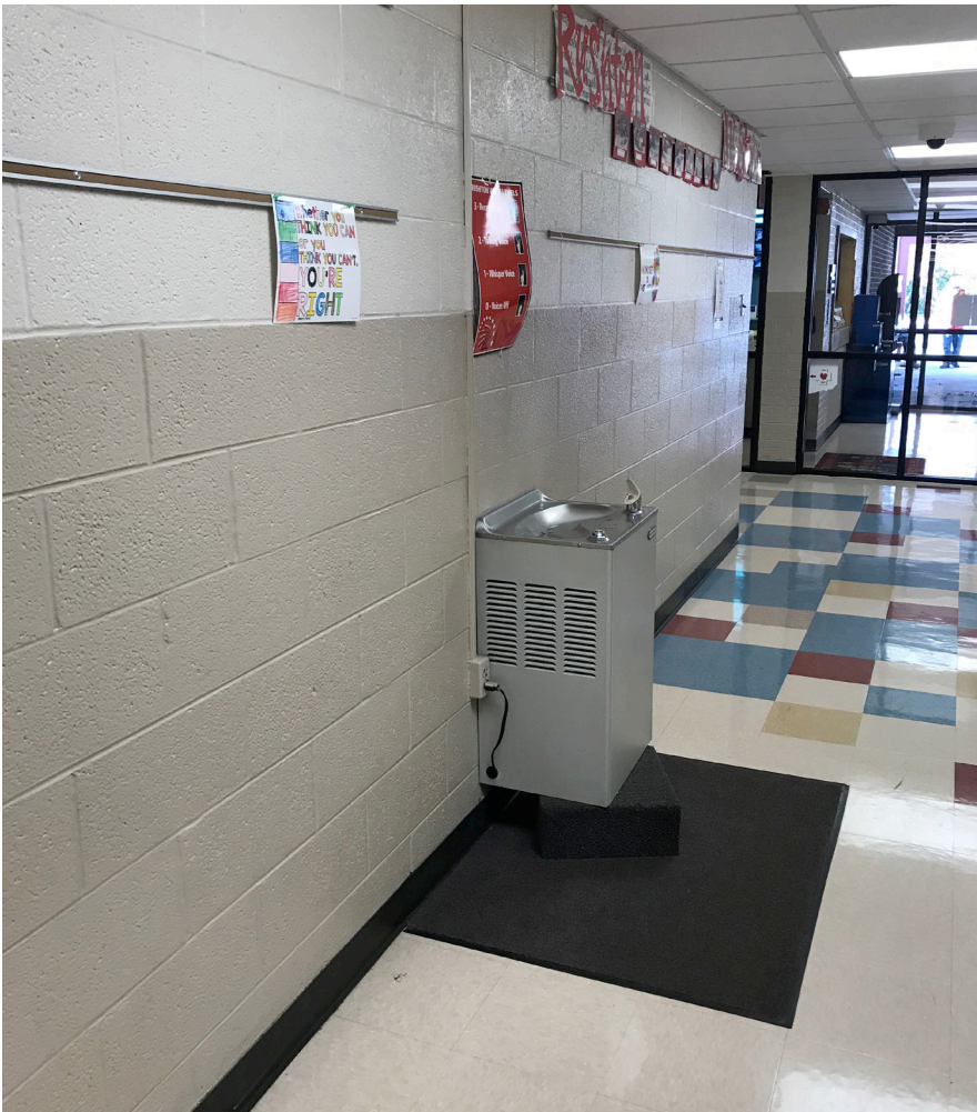
Drinking fountains protruding into Corridors more than allowed by ADA.
