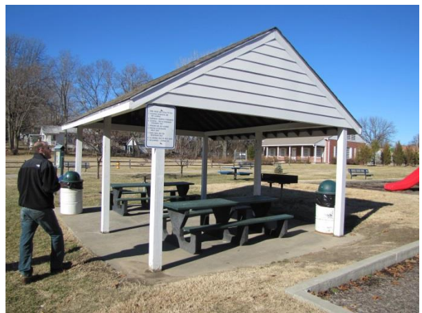
Image 4: The shelter provides a good gathering space, but is in need of maintenance. The open play field provides a good location for local residents in the surrounding neighborhood to hold practices and gatherings.
