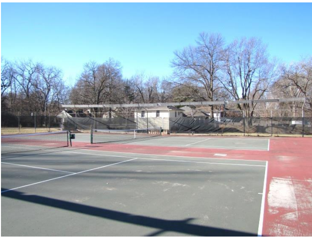
Image 1: The two tennis courts on site are in need of extensive repairs.
