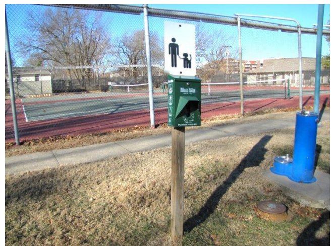
Image 4: Older sidewalks on site are in need of replacement and adjustments to meet accessibility standards. Additional connections are needed to drinking fountains, playgrounds and other site amenities.
