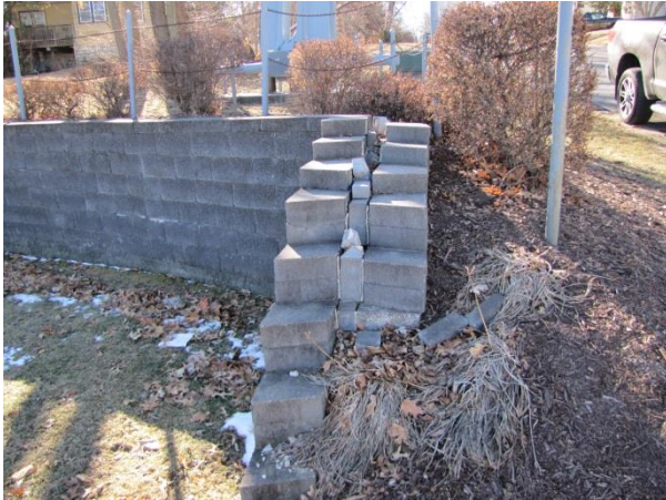
Image 1: The block retaining walls around the memorial site need maintenance.
