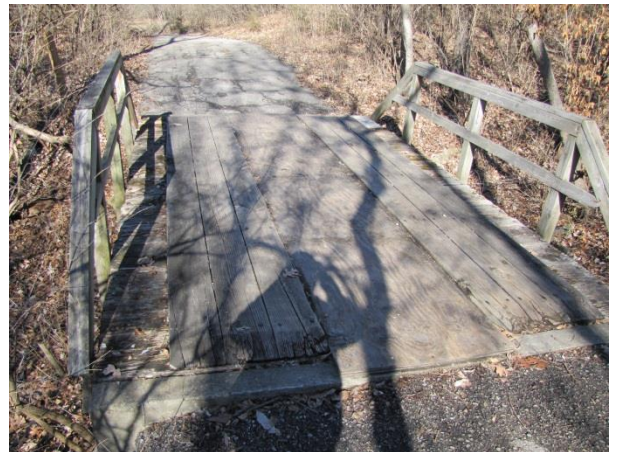
Image 2: The existing pedestrian bridge crossing has been temporarily patched; however significant safety concerns warrant full bridge replacement.
