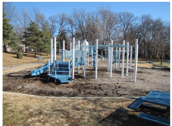
Image 4: Aging playground structures and surfacing are in need of updating to meet ADA standards.
